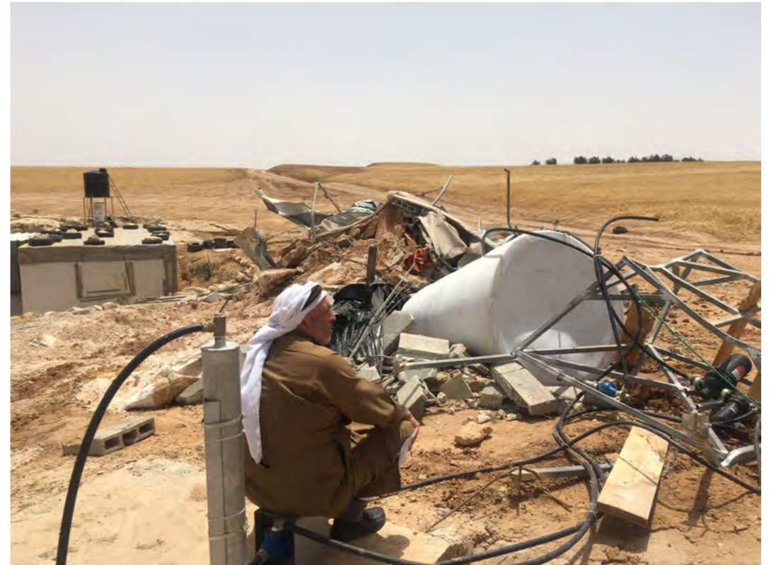
Al-Mirkez, Masafer Yatta, 918 Firing Zone, May 2, 2018. A man sits alongside the rubble of his home and a water tank following a demolition by the Israeli Civil Administration.
