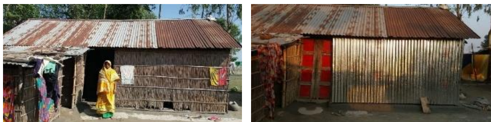
Picture taken by Sheikh Kamal: On the left one HH of Maiida Begum, before repairing, on right after repairing Katlamari village.
